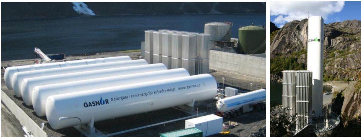
Figure 15 Horizontal and vertical pressurized tanks at Møsjoen (5000m 3 ) and Titania (250m 3 ), Norway. Source: Gasnor AS (Shell).
