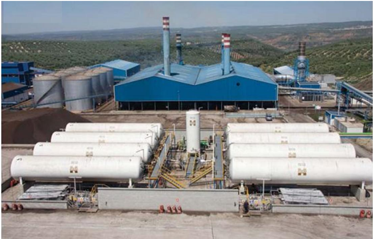
Figure 14 2000m 3 horizontal tanks in Jaen, Spain. Source: HAM Enagas.
